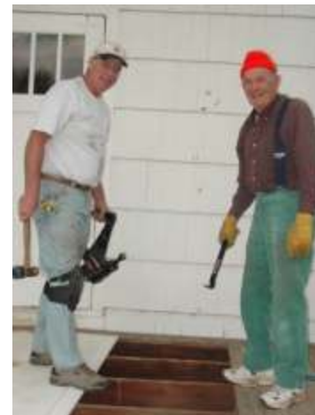
Replacing the Inpost Barn porch deck: Dale Kandel (left), Frank Hann (right). Thanks also to J.R. Schmucker & Doug Royar (above right).
